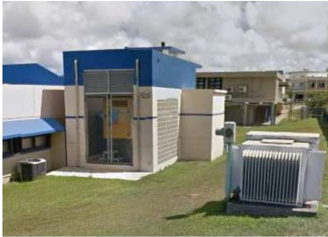
Backup generators, housed in structures similar to those at Buildings D (shown at left) and E, is a component of new construction projects together with power conditioners for A/C equipment and ew underground power service.
